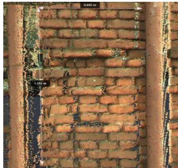
Fig. 9b. Washed-out bricks and mortar joint in the point cloud. The measurements are presented in the table
