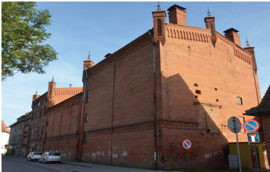
Fig. 5. The western façade with visible gaps
