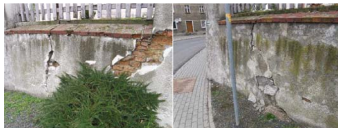
Fig. 8. Damage to the brick retaining wall (Bajno, 2014, photo by D. Bajno)
