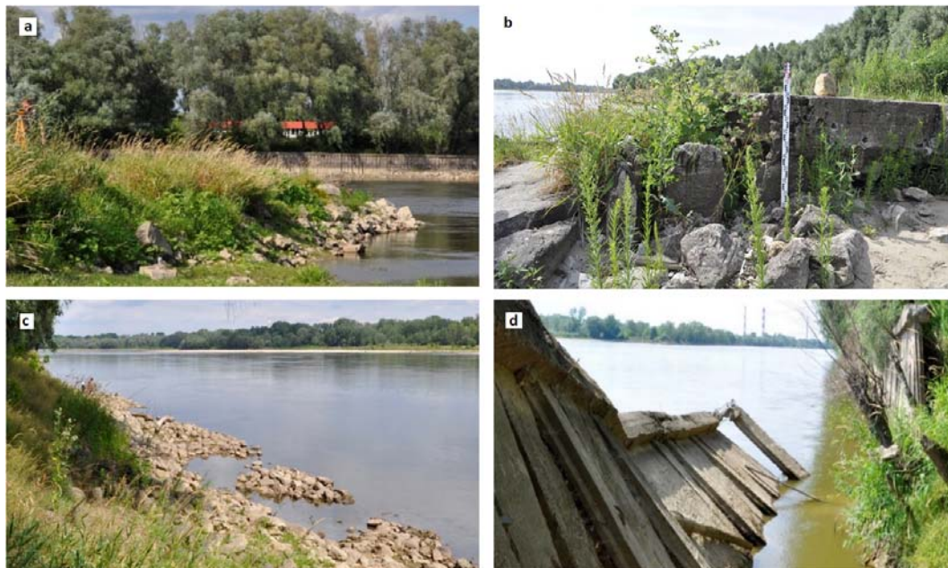
Fig. 6. River engineering structures (Kuźniar et al., 2017): a – left bank groyne, about 501.50 km, loosened stone riprap and irregular shape of the structure; b – left bank groyne, about 506.50 km, fault in the concrete body of the structure measuring approximately 80 cm, concrete slope facing destroyed; c – left bank protection, about 504.50 km, loosened stone riprap and sliding of loose boulders; d – right bank protection wall, about 501.40 km, loss of stability of segments of the concrete sheet pile wall
