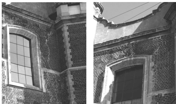
Fig. 19. Traces of repair of facade masonry of "old" Cathedral (photo by author)
