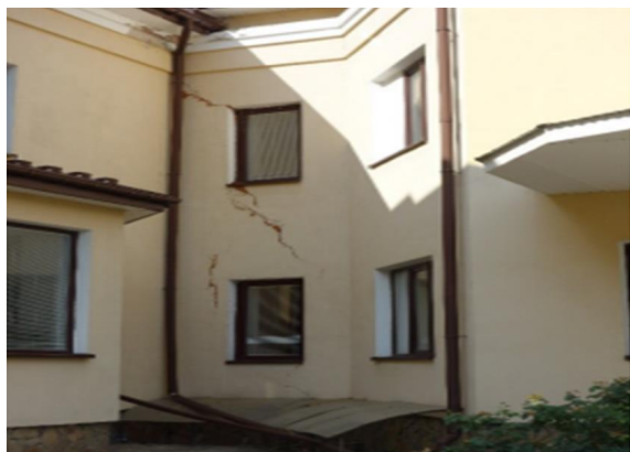
Fig. 3. Cracks/collapse on the external wall of the staircase at the multi-storey building at Port Harcourt (photo by the author)
