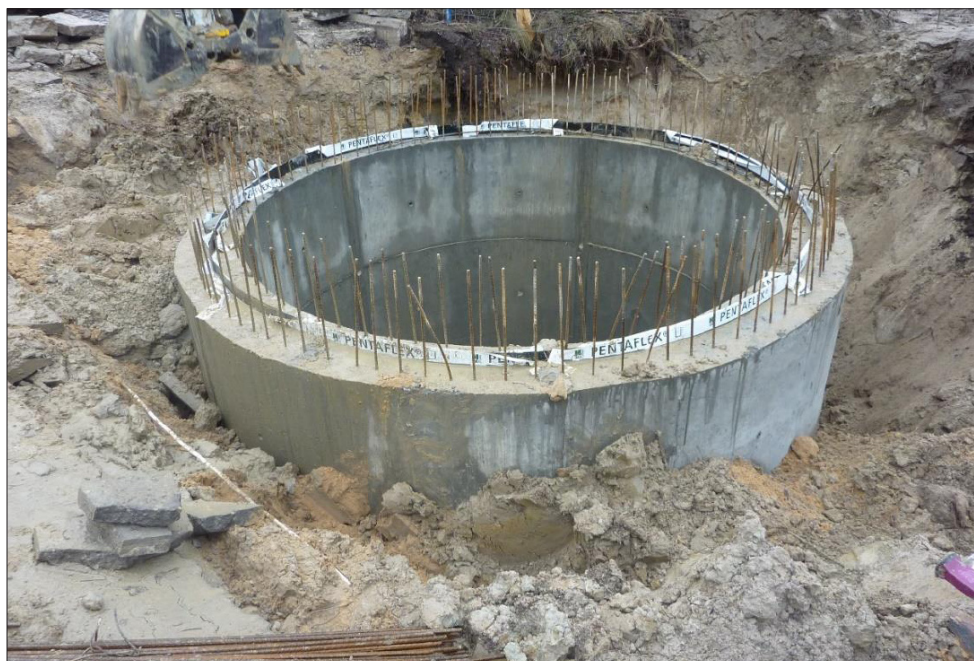
Fig. 11. Construction works on sinking the well in Suchy Las (the author's photo)
