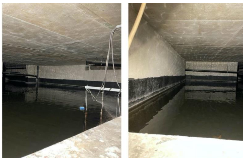
Fig. 3. Rainwater harvesting tank under the Sfera II Shopping Centre (photos by A. Boas Berg, 2018)
