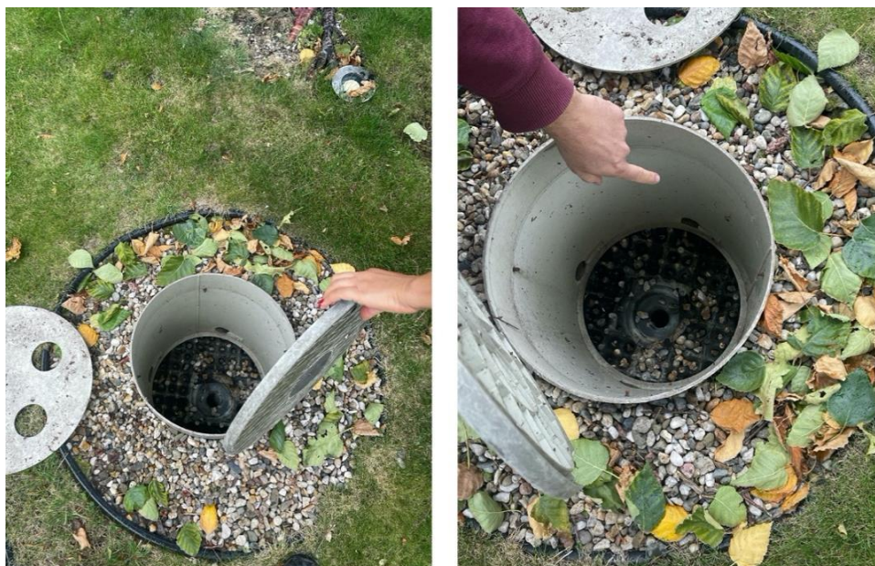
Fig. 6. The water drainage system on Sfera II Shopping Centre (photos by A. Boas Berg, 2021)
