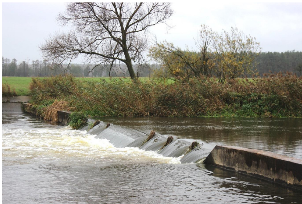
Fig. 5. Remains of the old impoundment on the Radomka river (photo by M. Kiraga)
