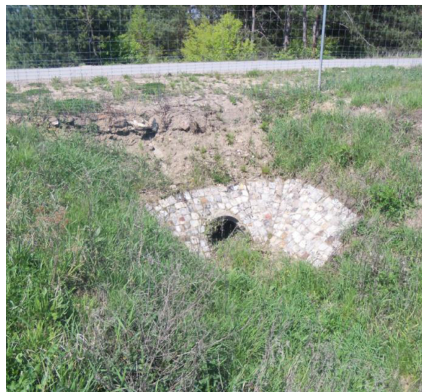
Fig. 9. The partly reinforced outflow. The lack of the full causes silting of the outlet
