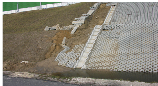
Fig. 1. Concrete reinforcement devastated by through flowing water from the slope
