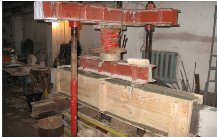
Fig. 5. Application of reinforce concrete jacket to the sample (final process of strengthening)
