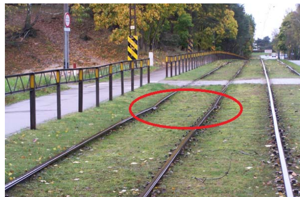
Fig. 3. Displacements of the sleepers in the track
