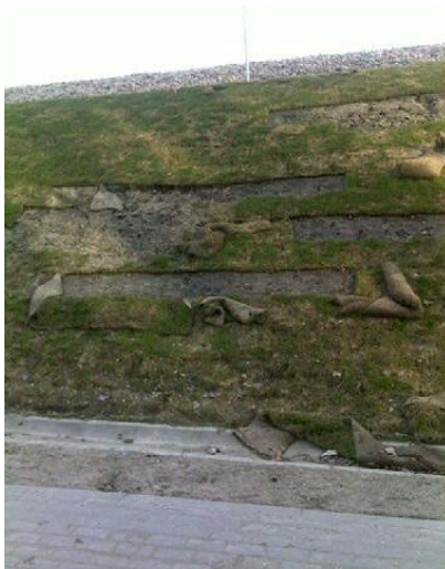
Fig. 2. Negative impact of the incorrect drainage on the condition of embankment slope (registered in March 2017)
