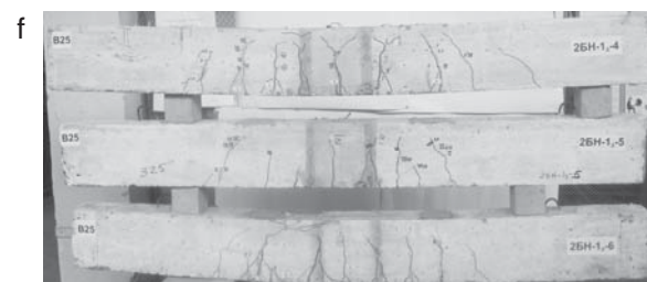
Fig. 4. The nature and location of the cracks in the tested beams: d, e, f – Concrete C20/25(B25)
