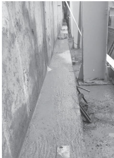
Fig. 12. Concreted reinforced concrete reverse transom along section C (41 running meter long) of the loading ramp retaining wall
