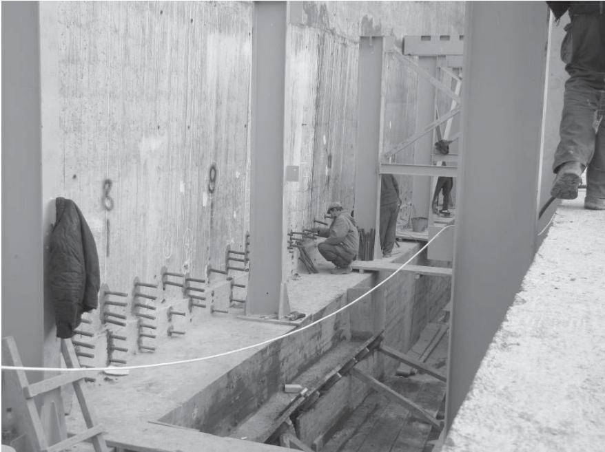
Fig. 10. Building in anchors \varnothing 32 mm into loading ramp retaining wall body with FIX-10M plugging cement
