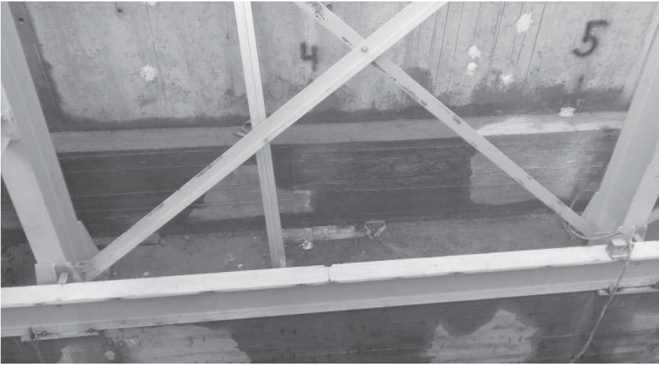
Fig. 11. External appearance of the section of the retaining wall reverse transom in the area of maximum crack openings (pos. 4–5) along the height of retaining wall reinforced structure
