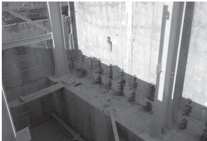
Fig. 9. Anchoring of the retaining wall reverse transom with reinforcement anchors Ø 32 mm A400C
