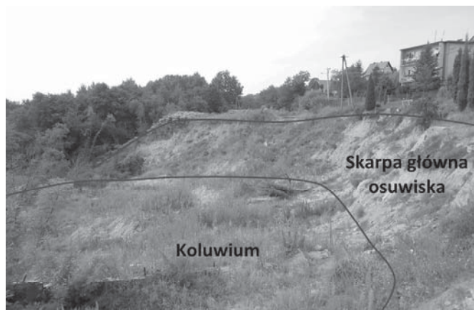
Rys. 1. Widok skarpy osuwiska Fig. 1. View of the slope of the landslide
