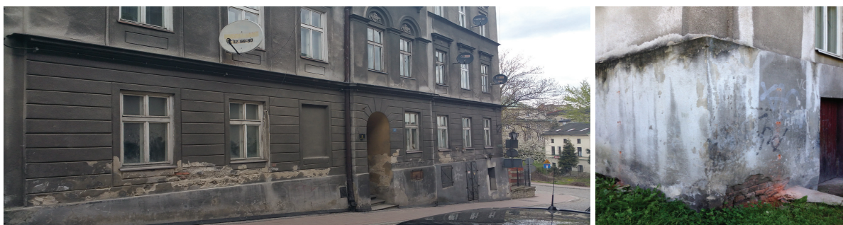
Fig. 4. House at 2 Waryńskiego Street, the figure shows the destruction of the walls caused by ground water rise
