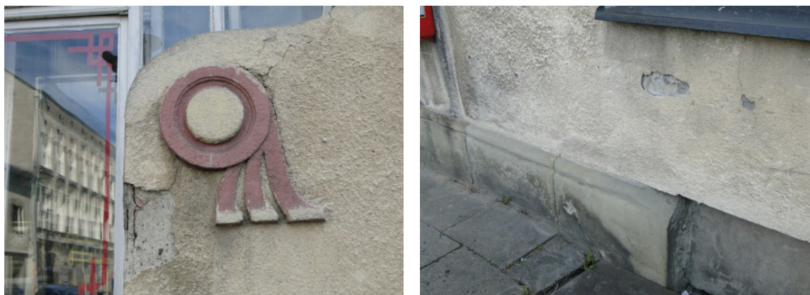
Fig. 2. Details of the facade of the “Under the Frog” tenement house at the Wojska Polskiego Square in Bielsko-Biała
