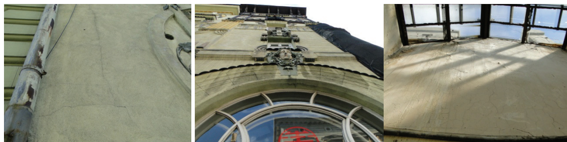
Fig. 3. Damage to the facade resulting from the impact of rainwater in the “Under the Frogs” tenement house in Bielsko-Biała
